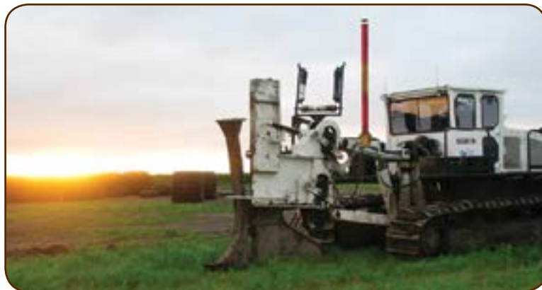
Tile plow. This is used to install the drain tile into the ground. Notice the rolls of drain tile in the background.
